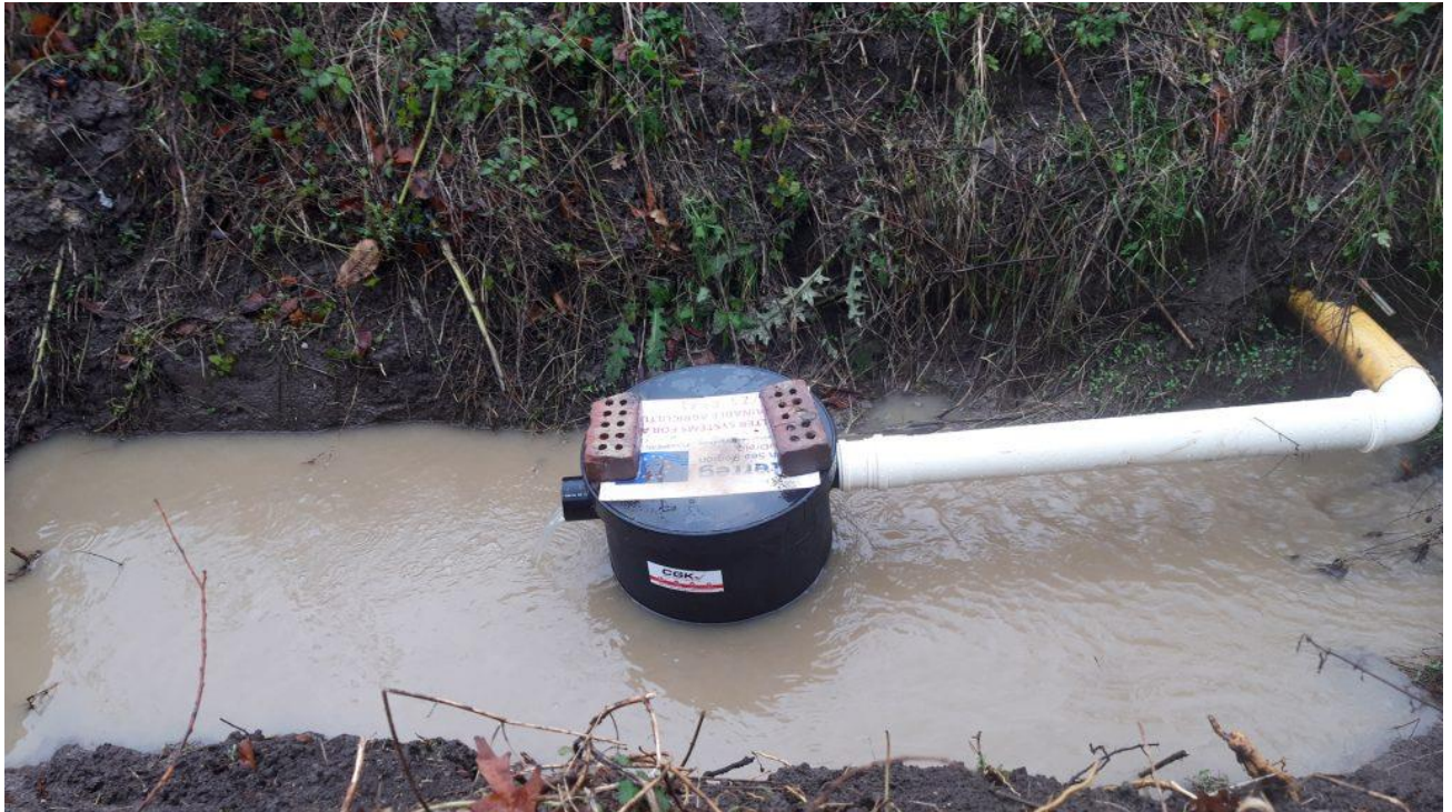
Fig. 1: A phosphorus filter box is directly connected to a tile drainage pipe. The filter box is filled with iron-coated sand (ICS), which adsorbs phosphate and lowers the phosphorus concentration in the ditch water.
